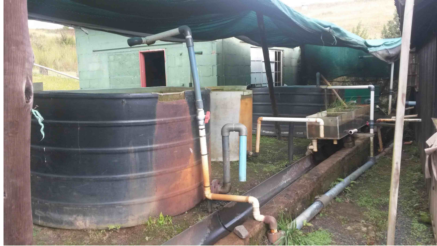
Figure 2.3: Mbona fry tanks are plastic jojo type tanks used for rearing the fry till they are old enough to move to the tanks. The flow rate through the tank is controlled by an inlet valve and the depth of water in the tank is determined by the height of the overflow outlet pipe.
